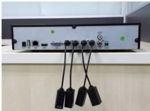
Old baluns make the cabinet a mess
